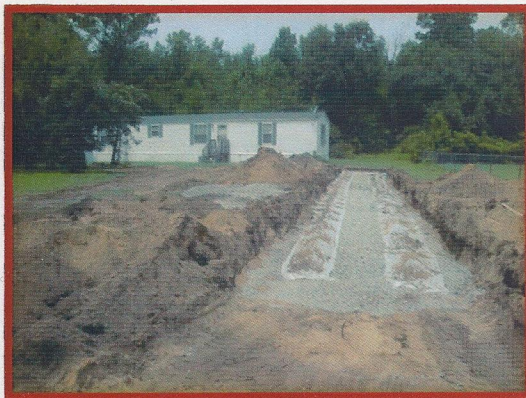
Grant-funded installation of a shallow septic system in the Sewee to Santee area
